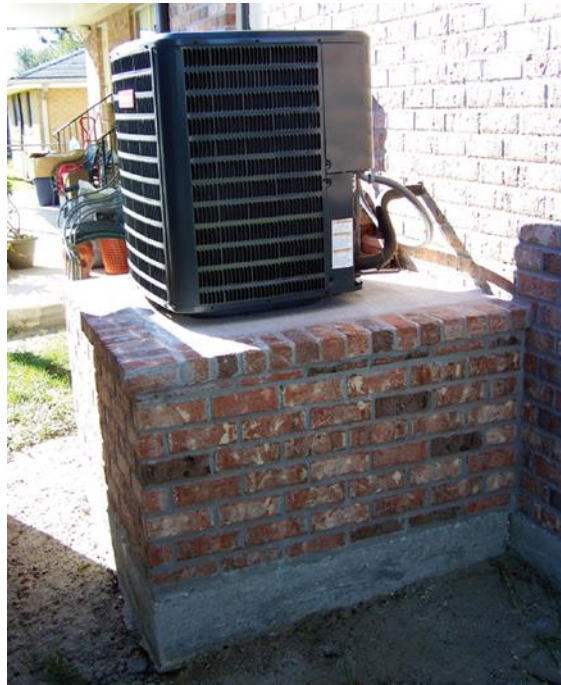
Figure 2-41: An example of an elevated air conditioning unit. (Source FEMA P-348 – Figure 3-1)
