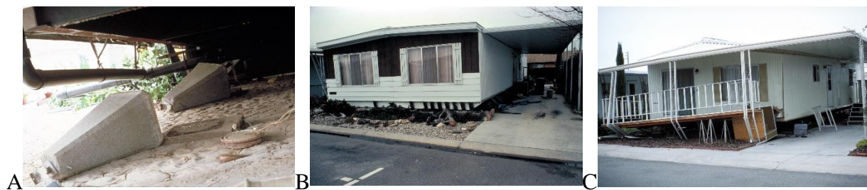
Figure 2-54: Earthquake damage to manufactured housing. (A): Overturned concrete piers that supported a manufactured house, viewed after the 1978 Santa Barbara earthquake. (B) and (C): Collapsed manufactured houses after the 1980 Livermore earthquake. (Images courtesy of National Information Service for Earthquake Engineering, University of California, Berkeley.)
