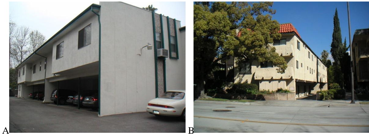
Figure 2-49: Soft-story wood-frame multifamily dwellings. (A) Menlo Park, California. (B) Pasadena, California. (Photo credit: Porter 2006, used with permission.)
