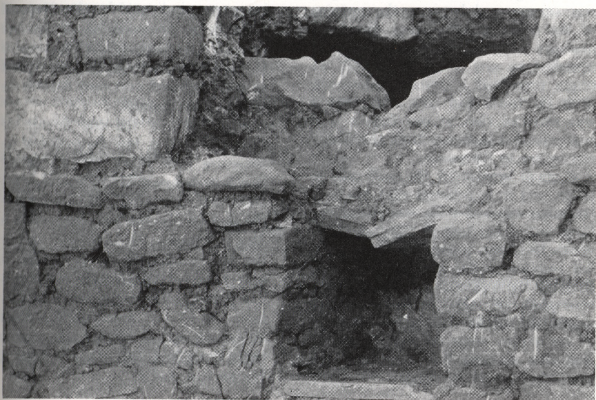
PLATE 16. Kiva B, Niche 3. Above it is opening to passage leading to Kiva A.
