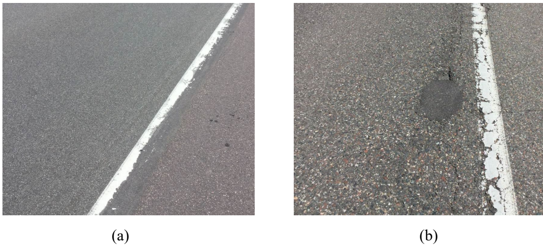
322 Figure 5: US-169 pavement surface showing locations with (a) low, and (b) high IRI values.
