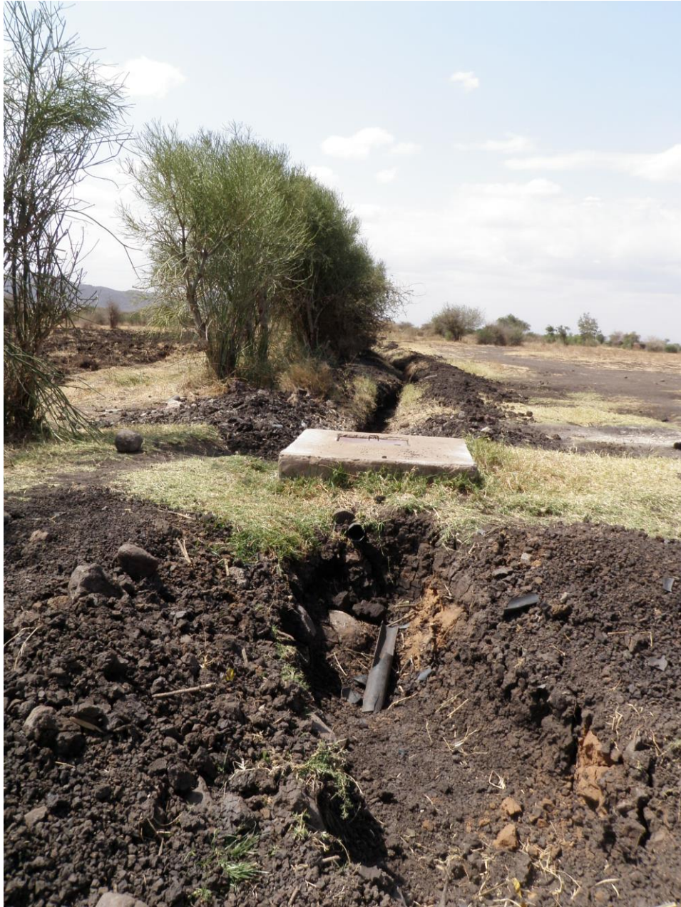
Figure 3. Irrigation pipes in Burat. (Photo credit: Amy Quandt, August 17, 2014)
