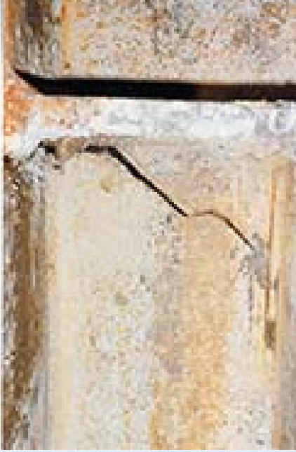
Figure 2. The 1994 Northridge earthquake revealed fragility in the welds that connect beams to columns in a kind of steel frame construction commonly used in tall buildings for the previous few decades. This figure shows an actual fracture observed in a building after the earthquake. Photo by J.C. Anderson, 1994, from the Earthquake Engineering Online Archive NISEE e-Library, UC Berkeley, with permission.
