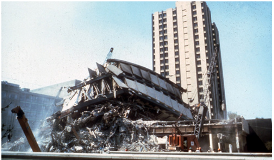
Figure 1. Collapsed steel-frame Pino-Suarez Towers after the July 28, 1985 Mexico City earthquake. A 14-story building collapsed on top of an adjacent one. Photo by E.V. Leyendecker, UC Berkeley NISEE e-Library, with permission.
