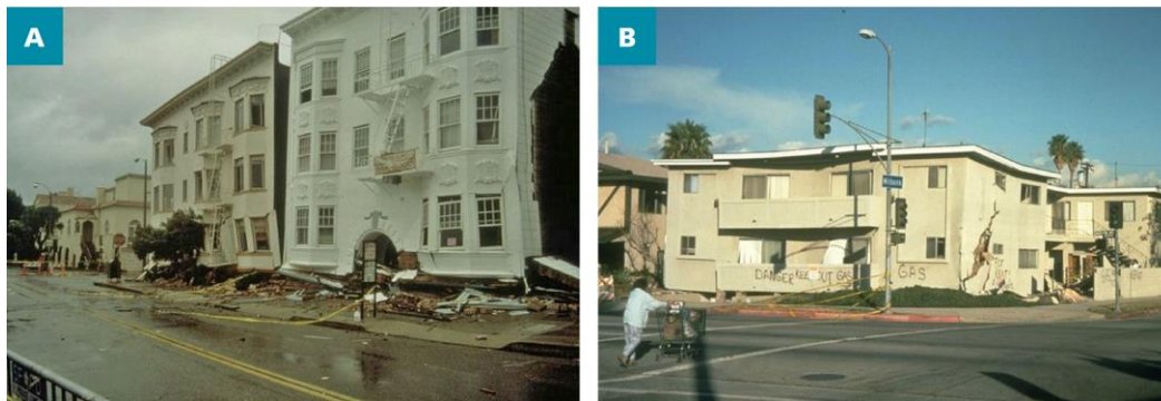
Figure 1. Collapsed soft-story wood-frame multifamily dwellings in (A) San Francisco, 1989 Loma Prieta earthquake (B) Los Angeles, 1994 Northridge earthquake
