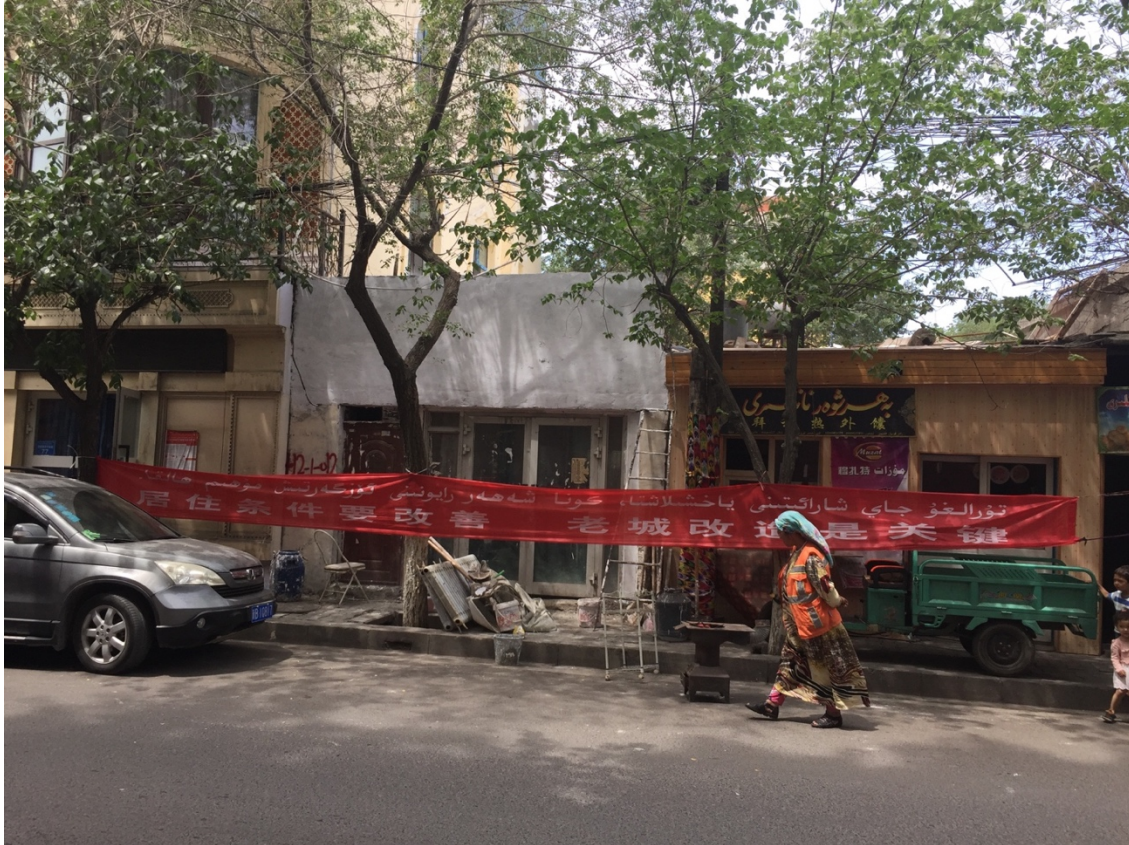
Figure 5.3: In May 2017, Demolition occurred on 90% of Uyghur streets and businesses. This once-lively business district sits empty the day after the in the area shops were forcibly closed. The propaganda banner reads: “The residents’ living conditions must be improved; Old city redevelopment is crucial” (居住条件要改善；老城改造是关键). Source : Photo by author, May 2017.
