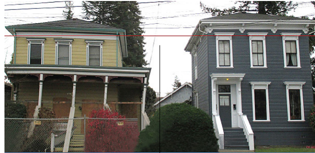
This house was not retrofitted and slid off its foundation in an earthquake
