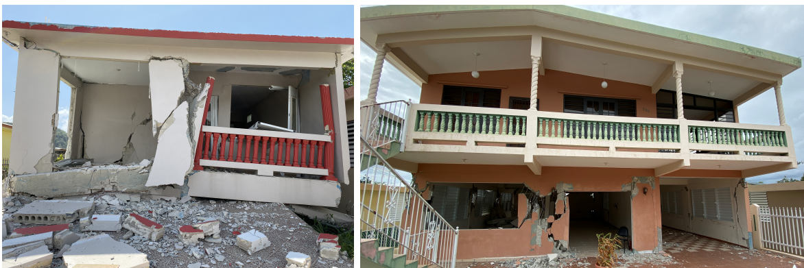
Figure 3.2: Damage to RC houses in Guánica with (a) an open ground story, showing loss of the first open story, and (b) masonry walls between columns at the first story, showing shear cracking in walls and columns. [Photos: Polly B. Murray]
