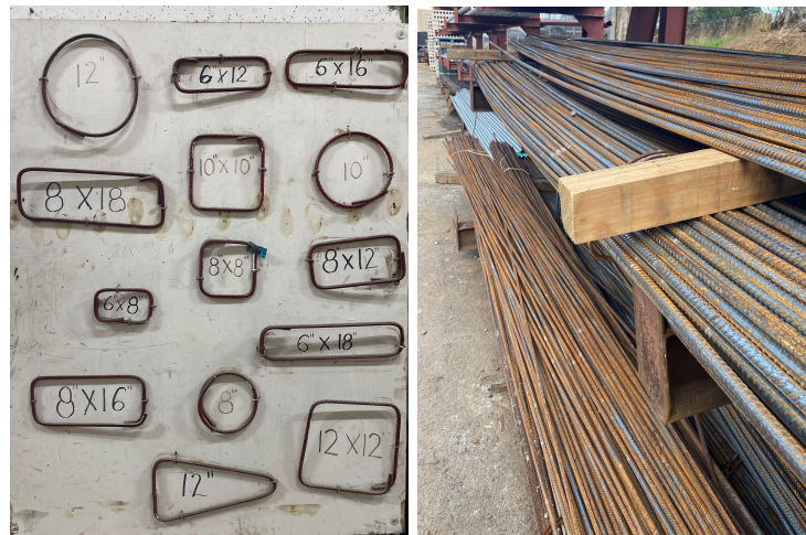
Figure 3.11: Steel reinforcing bars used in home construction. Transverse ties are sold in pre-defined bent shapes; the 6 x 12 in bars are most common. The most common longitudinal bars are no. 4 and no. 5, and are often stored outside (Humacao, Puerto Rico). [Photos: Polly B. Murray]
