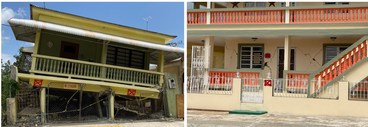
Figure 3.7: Houses in Guánica that were damaged during the January 7, 2020 earthquake. (a) failure in first story columns, (b) shear cracks in masonry walls. [Photos: Polly B. Murray]
