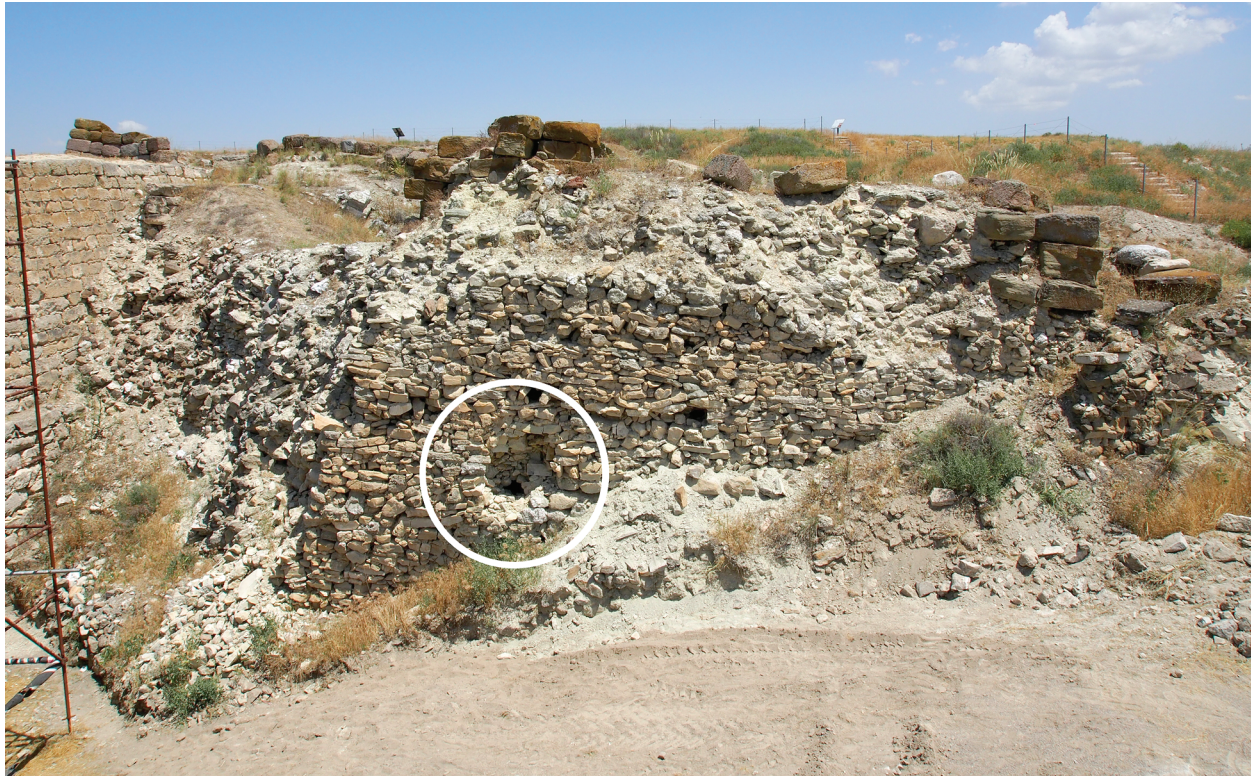
Fig. 19. View looking north toward the rubble fill: The circle indicates the location of the 2015–2016 collapse in the main face of the rubble. At the top above that area are the precariously situated blocks of the North Court of the Middle Phrygian Gate. To the left is the too-steep rubble slope resting in part against the east outer wall of the North Bastion of the Early Phrygian Gate Building. (Photo by S. Gönen)
